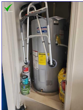
The Water Heater Area
