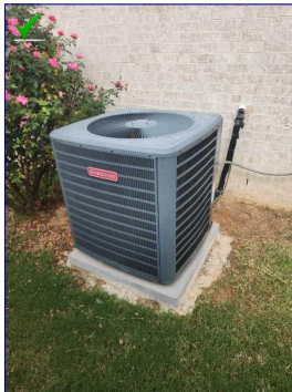
The air conditioner compressor/condenser
