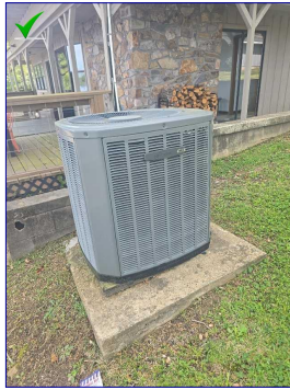
The air conditioner compressor/condenser.
