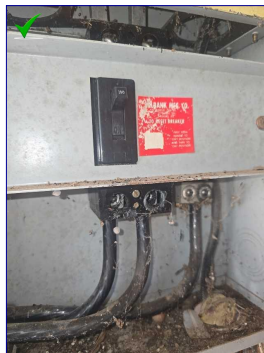
The main electrical service panel
