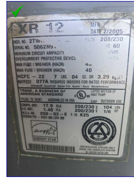
The air conditioner compressor/condenser data plate. 2005 year. Appears to be a 3 ton unit.
